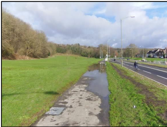
Photograph 5.8: Ponding on footway adjacent to Wild Park
