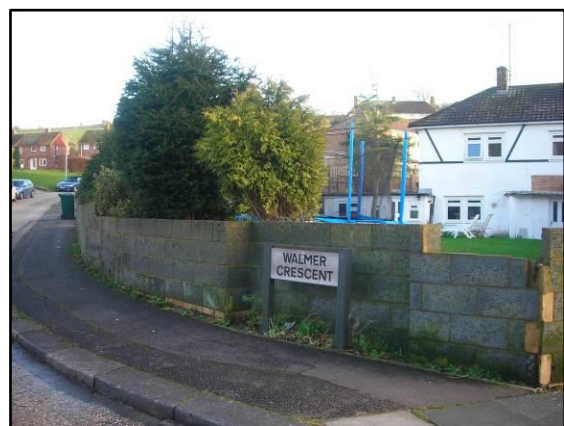
Photograph 5.13: Wall acting as flood defence structure
