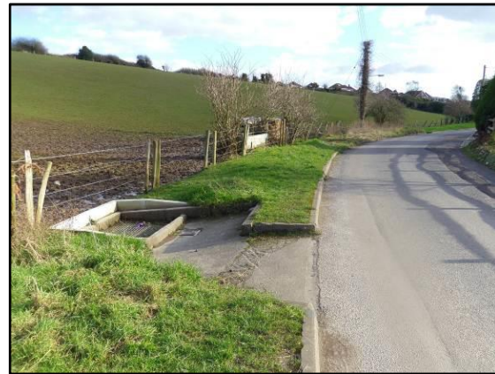
Photo 5.35: Super Gully and saturated ground
