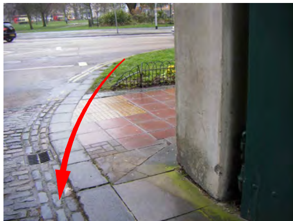
Risk to pedestrians, soft landscape and stonework from larger vehicles cutting the corner.
