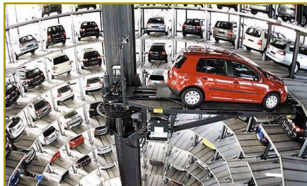
Hi tech parking system Volkswagen, Wolfsburg, Germany
