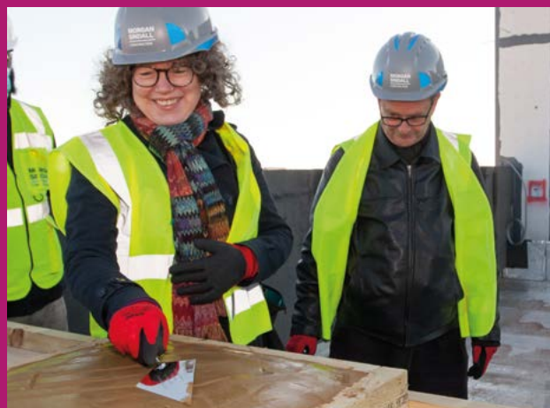
Councillor Siriol Hugh-Jones and Councillor David Gibson at the 'topping out' ceremony of the development of new council-rented homes in Victoria Road, Portslade.
