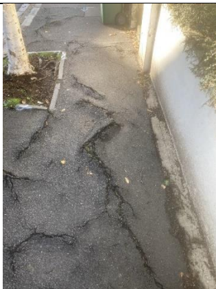
Tree Root Damage
