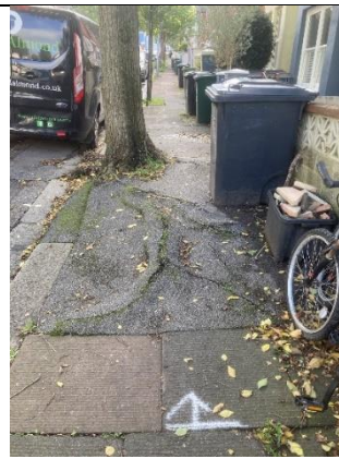
Tree Root Damage
