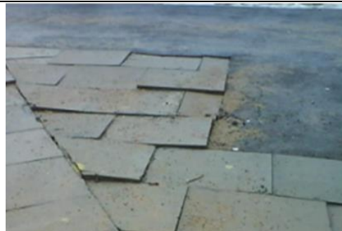
Uneven Flags/abrupt-level difference
