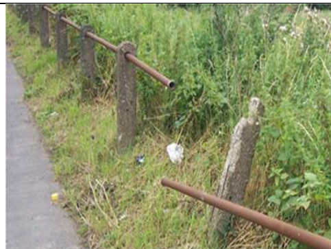
Damaged Fence (pole projecting into the highway)
