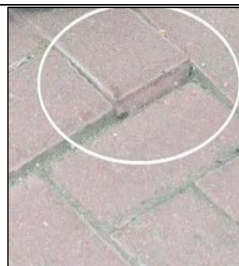
Paving Block Abrupt-level Difference
