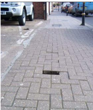
Missing Paving Block
