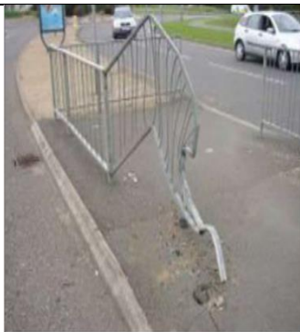
Damaged Pedestrian Barrier (at ped crossing location)
