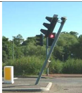
Leaning Signal Pole
