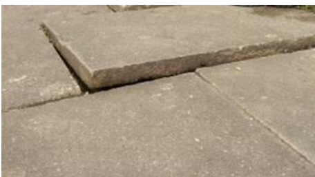
Uneven/Unstable Flags/abrupt-level difference
