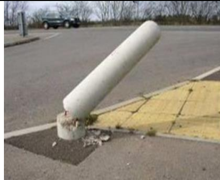
Damaged Bollard (overhanging Tactile Paved Crossing)
