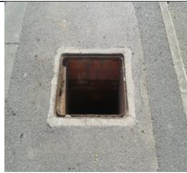
Missing Utility Cover
