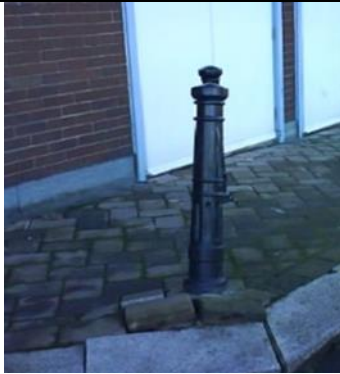
Damaged Bollard and Displaced Block Paving
