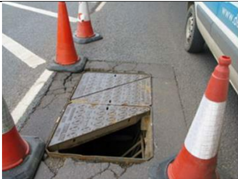
Missing Utility Cover
