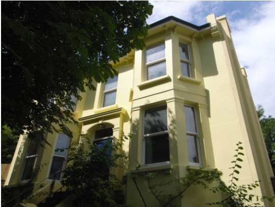
Example of 'hybrid insulation': external wall insulation is installed on the side and rear of the property, and internal wall insulation is fitted internally on the front wall. Image: Low Carbon Trust
